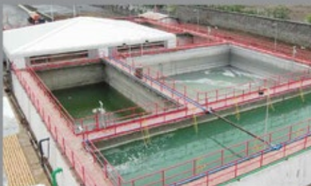
Fiat India Automobiles Effluent & Sewage Treatment Plant, India
