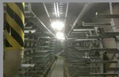
Prague City Utility Tunnels, Czech Republic
